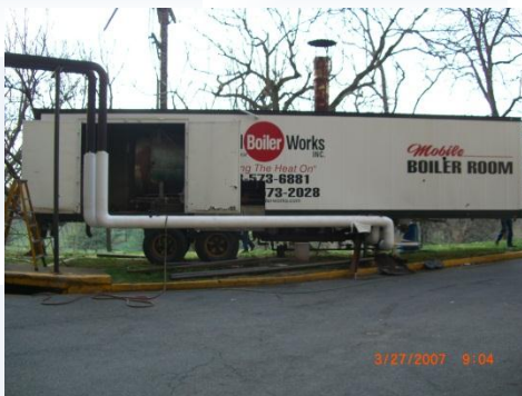
Rental Boilers, Chillers, and DHW Systems
