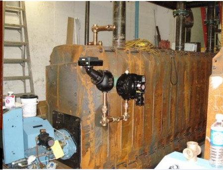
Cast Iron Boiler Installations
